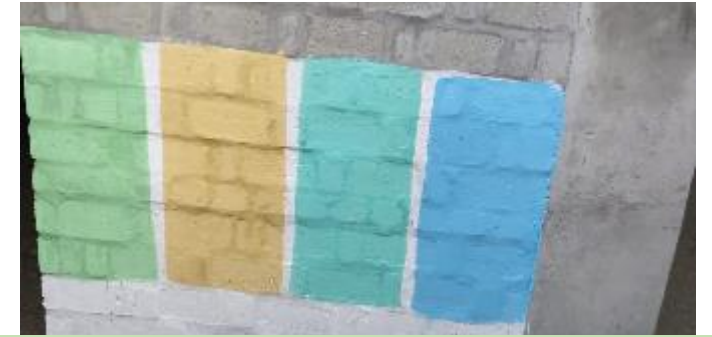
Sample painting done in outer wall using Prakritik Paint. Second colour from left is selected by HMRD
